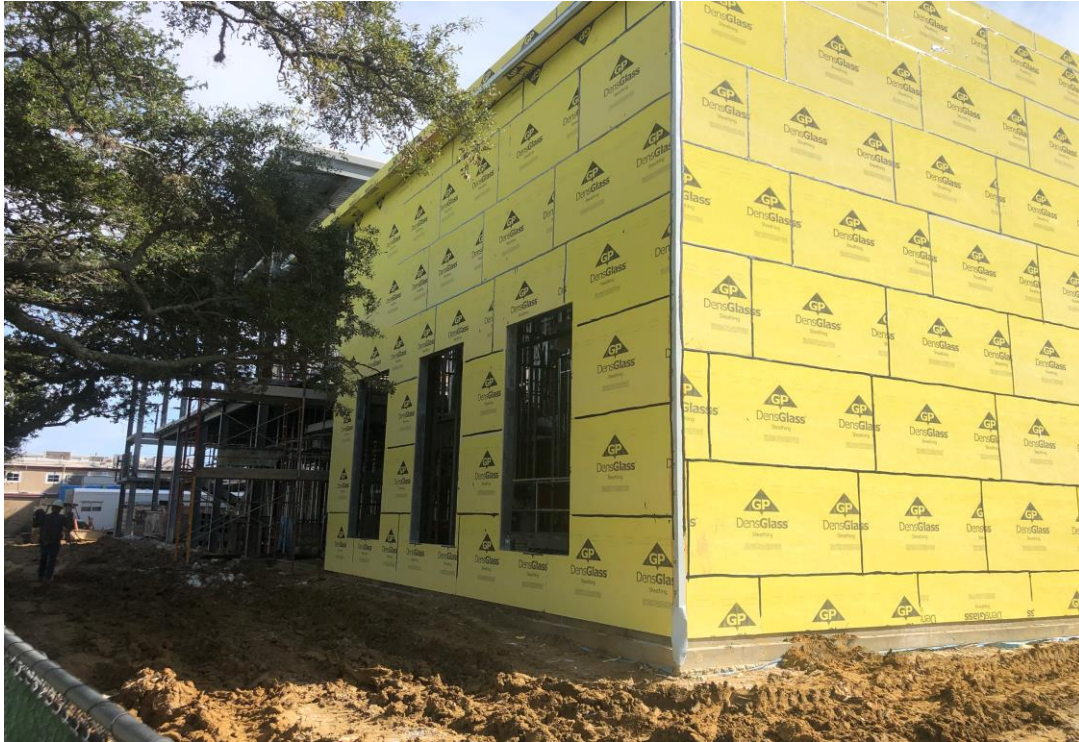
Exterior sheathing installation is underway at the Band Hall area at Lee High School
