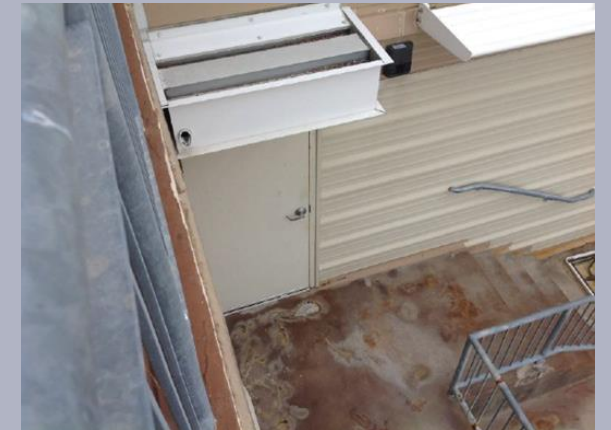
Failed membrane at press box
