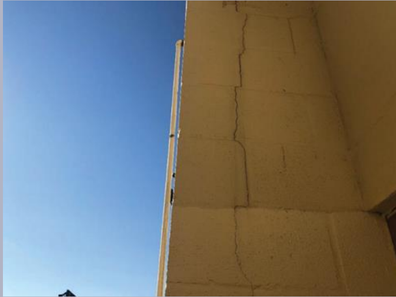
Damaged CMU walls
