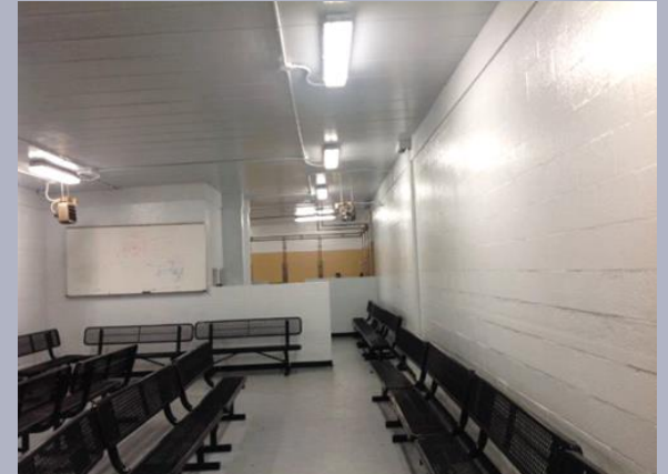
Various issues at locker rooms
