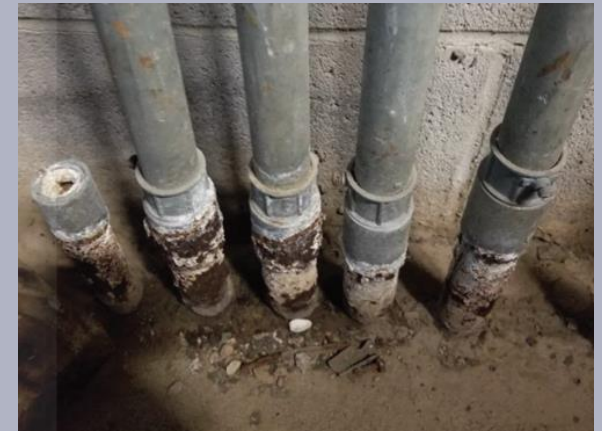
Deteriorated steel conduit
