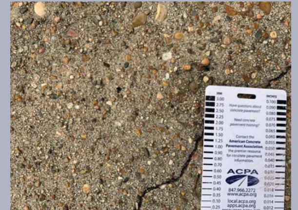
Cracks on ramps
